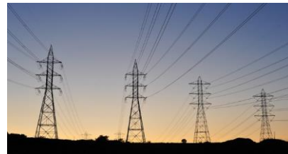
Power plants connected to the grid
